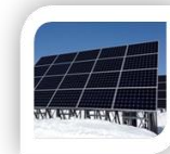
Location: Hokkaido Size: 1.2MW
